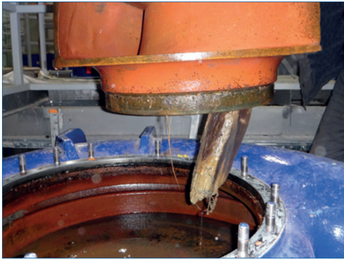
Fig. 91: Wood inside the impeller of a KRT pump
