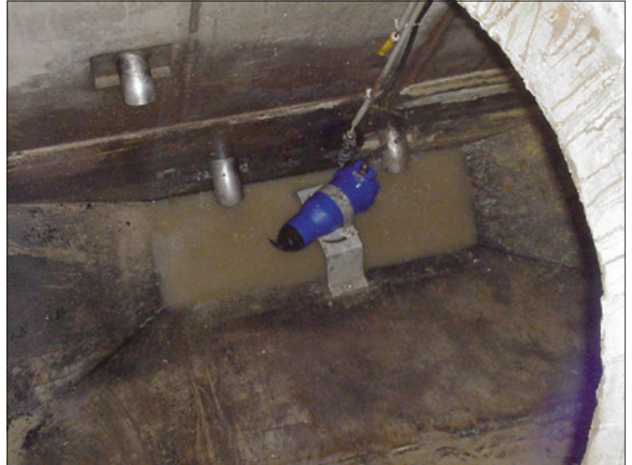
Fig. 103: Submersible motor mixer in the pump sump
