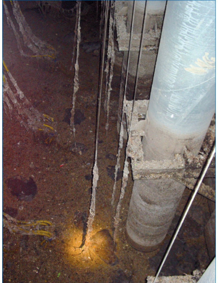
Fig. 92: Formation of a layer of scum in the pump sump
