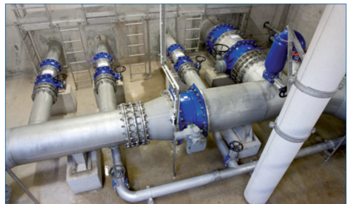
Fig. 55: Valve chamber with the piping integrated horizontally
