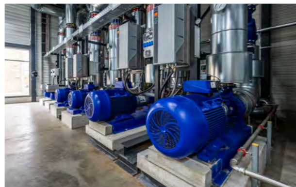
Reliable and efficient: KSB pumps in a biomass power plant
