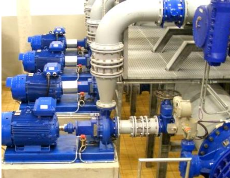
Figure 5 Four of eight parallel PaTs in service at the water utility authority (Zweckverband Landeswasserversorgung, Stuttgart, Germany) in Stuttgart
