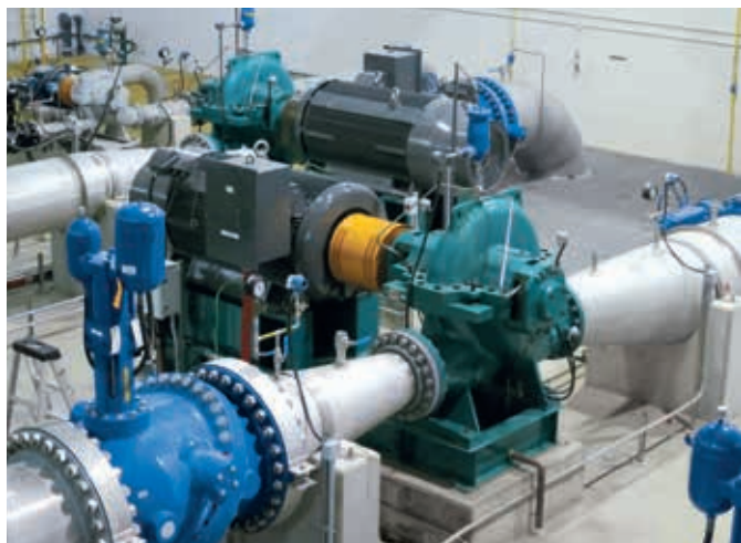
Airport Road Pumping Station
